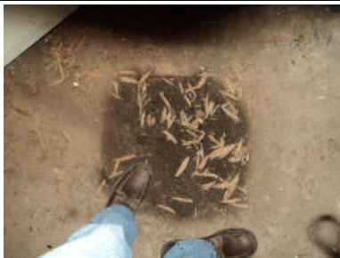
Appears functional. Drains are not tested.
