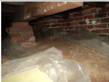
Vapor barrier needs to be straightened out.
