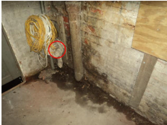
The old sink drain is not properly capped off.
