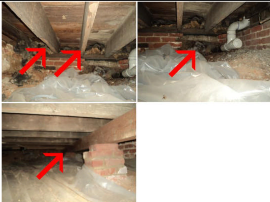
Evidence of past insect damage to the joists under the front foyer. Recommend sistering these joists. There is a large opening in the front foundation wall under the front door. Evidence of past repairs to the floor joists under the living room.
