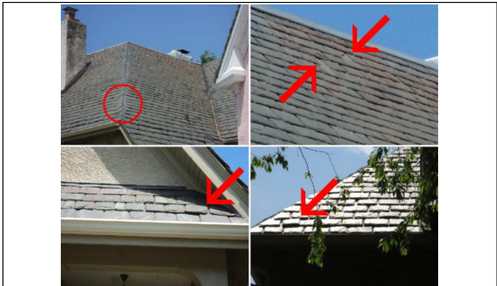
Some of the ridges need to be sealed. There are a few damaged and loose slates visible. There is a loose flap on the flat roof over the rear porch.
