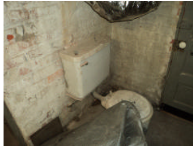
The toilet is no longer in use and should be capped off to prevent the trap from drying out.
